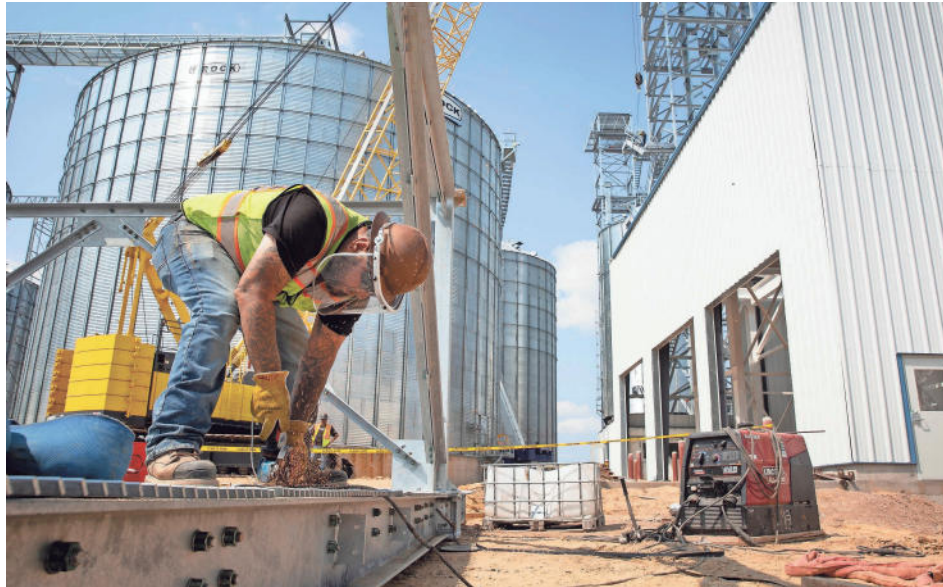
Crews from Mid-States Millwright & Builders work on rebuilding damage at Key Cooperative near Marshalltown, Iowa. The location was one of many the organization lost to the Aug. 10, 2020, derecho that swept through the Midwest.
