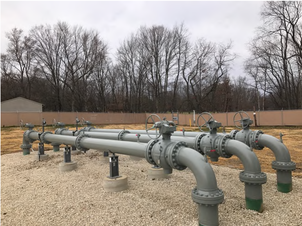
EXAMPLE OF METERING STATION
