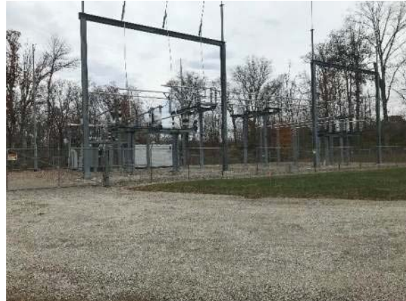
Photograph 10: Looking east towards Str. HL903 and substation beyond. (November 14, 2018)
