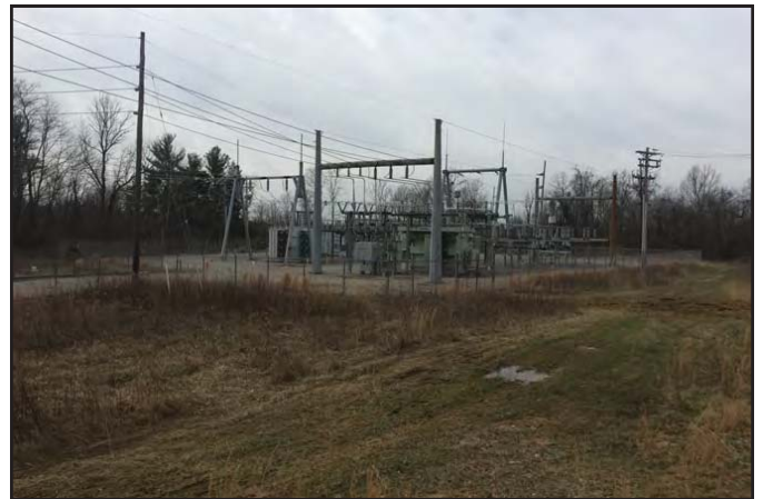
Photo 8: View of the existing substation.
