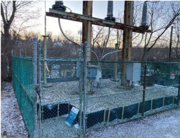
Photo 4: Existing substation, Looking SE
