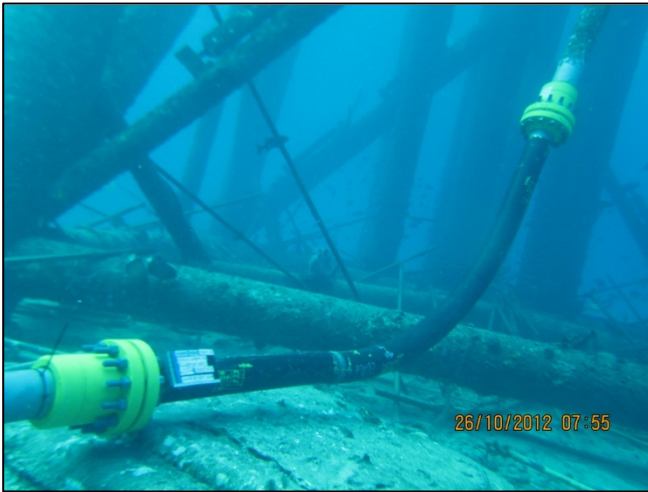
Figure 6: Replacement of 20D Riser Bottom Bend to allow for smooth RTP Pull-thru
