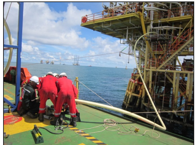
Figure 11: Splice Coupling Tail of Pipe
