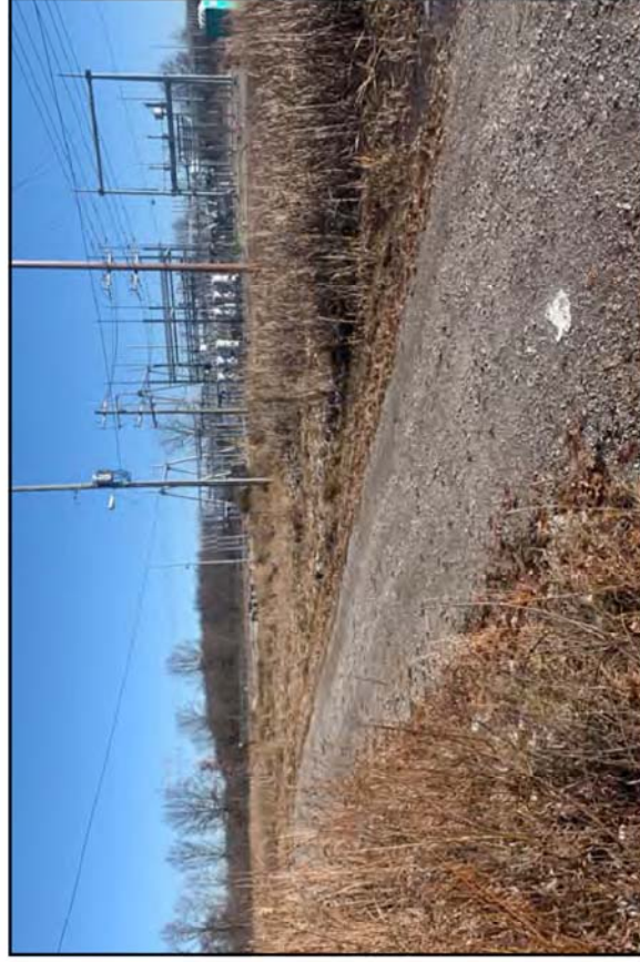
Photo 4: Duke Energy Substation, impervious surface.
