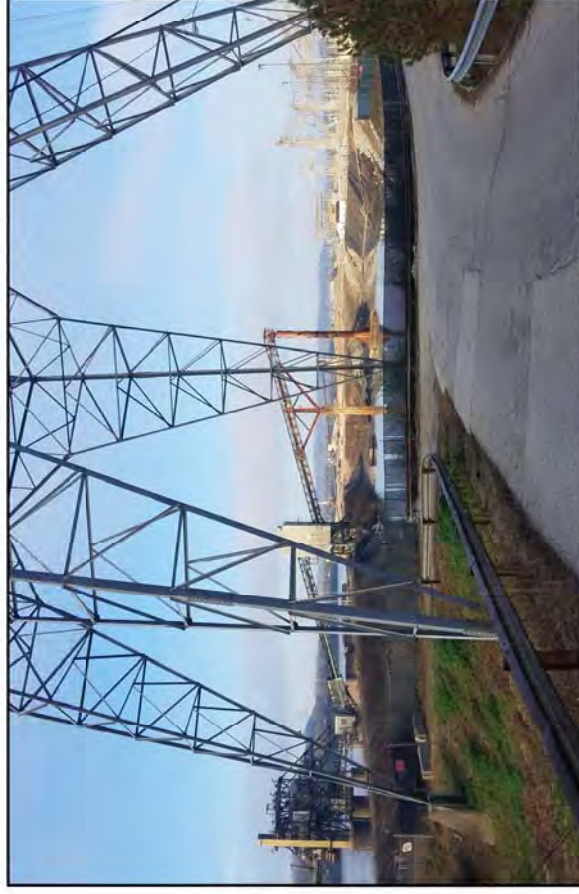
Photo 4. Duke Energy Structure 6BN-X31-2, View Looking Southwest, 04/02/2020.
